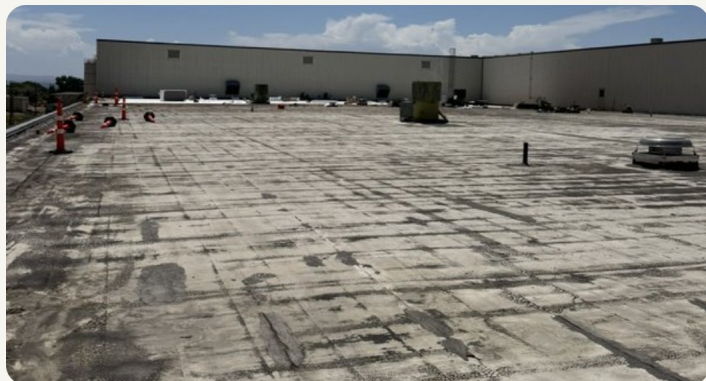
Before: worn, cracked roof surface.
